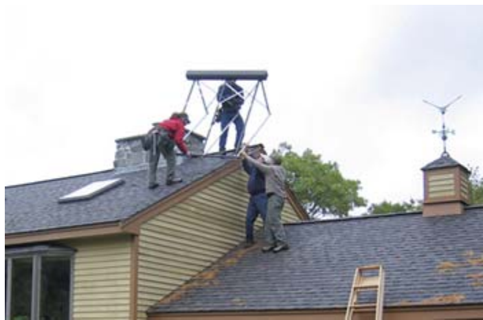
An “energy raiser” in action. PAREI members pitch in to install a solar water heating system.
